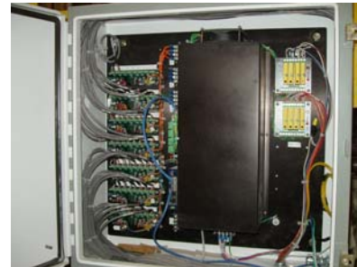
Data Concentrator adjacent to sensor array collects data and transmits to PC
